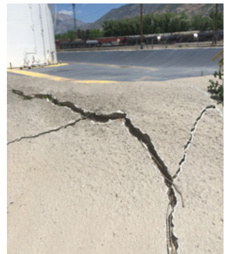
Example of an out-of-compliance berm.
