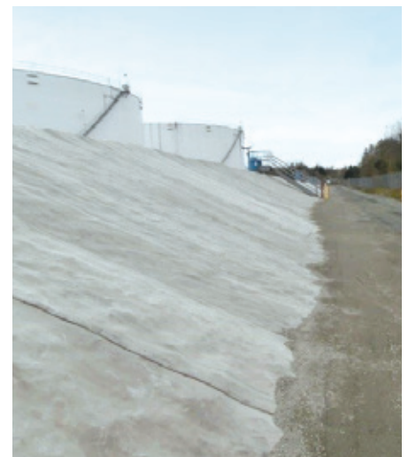
Required permanent engineered barrier around terminal storage tanks.
